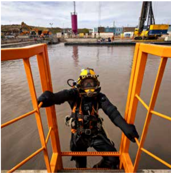
A diver inspects the quality of works in the pit of the PALLAS-reactor
