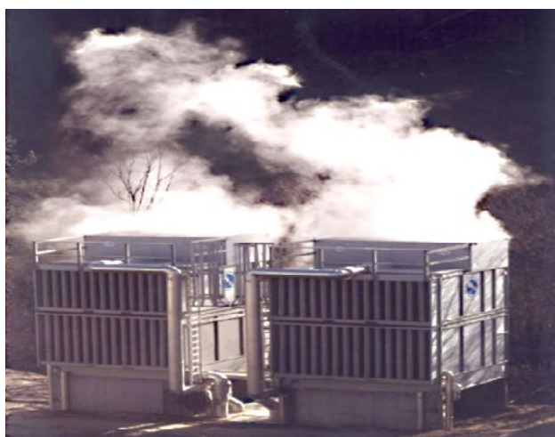
Figure 63 Reference condensation formation of cooling installation
